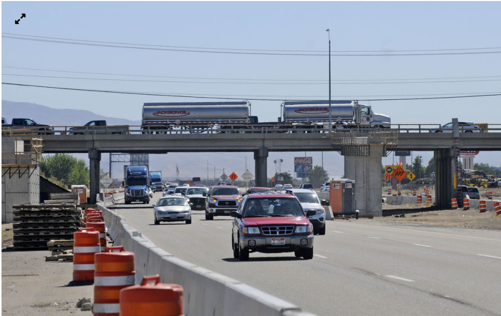
Vehicles pass under the Meridian Road Interchange on Interstate 84 during the interchange rebuild in 2014.
