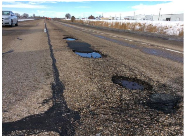
Numerous potholes received emergency repair starting Jan. 11 from the Idaho Transportation Department along Interstate 84 between Nampa and Caldwell.
